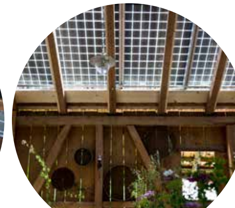
2013 / Scheune GS-Module / 14,04 kWp
