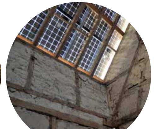
2011 / Scheune GS-Module / 13,72 kWp
